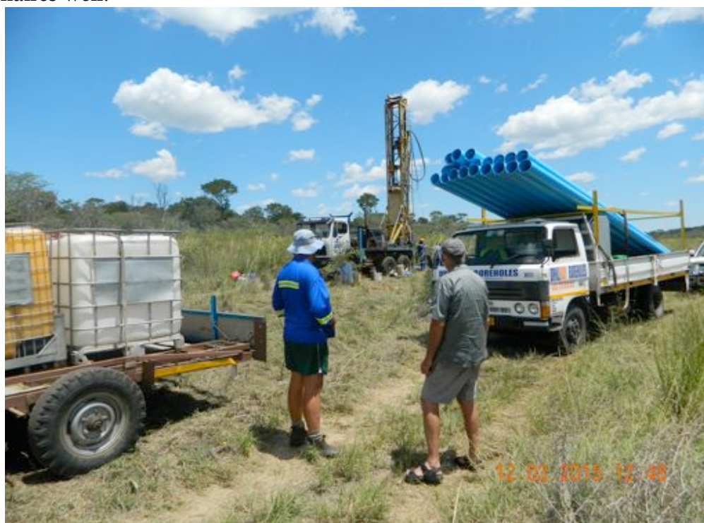
The first borehole going in on the Mabuza Vlei – Unit 7. Good water found
